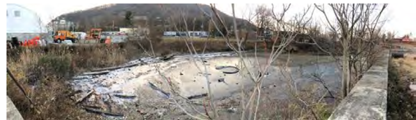
Debris and Siltation at Fowler's Gap Outfall
