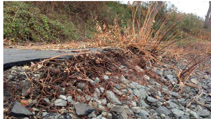
HHQP pathway erosion damage after Hurricane Sandy
